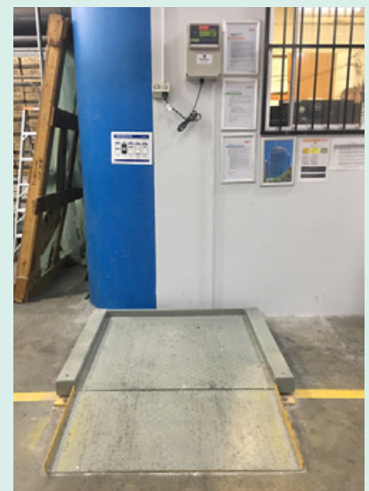
Weighing device in the loading dock, providing quality secondary source of waste data
