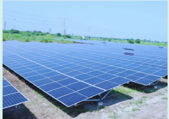
CLINT's captive solar plant in Tamil Nadu will generate the power supply needed for 2 million sq ft equivalent of office space
