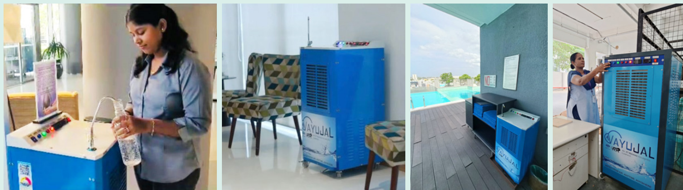
AWGs placed in four key high-traffic areas — the lobby, banquet hall, gym/swimming pool, and at the staff entrance
